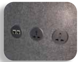
AH Meyer Power & RJ45 Data Point
